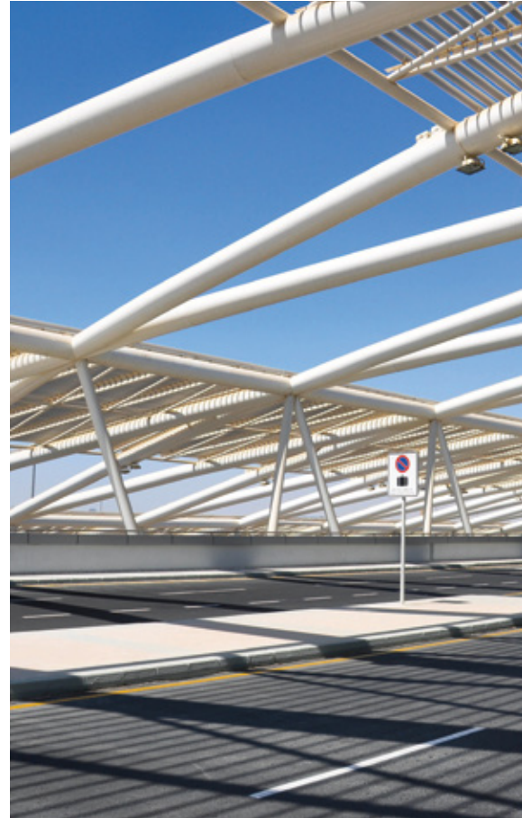
Cairo International Airport, Terminal 3 – protected by SteelMaster
